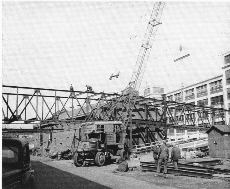
This covered ramp, under construction, when finished will connect Buildings 109 and 112 with Building 140, and the receiving and shipping rooms of that building. Materials shipped in or out of 109 and 112 will, thus, be given an under-roof connection with rail. The overhead bridge will also provide under-roof travel for employees.
